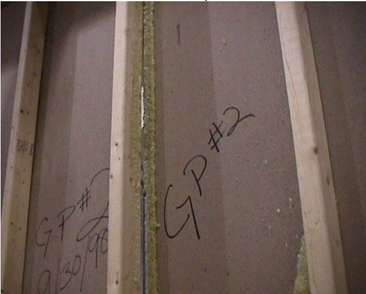
Test No. 2 at Failed Area
