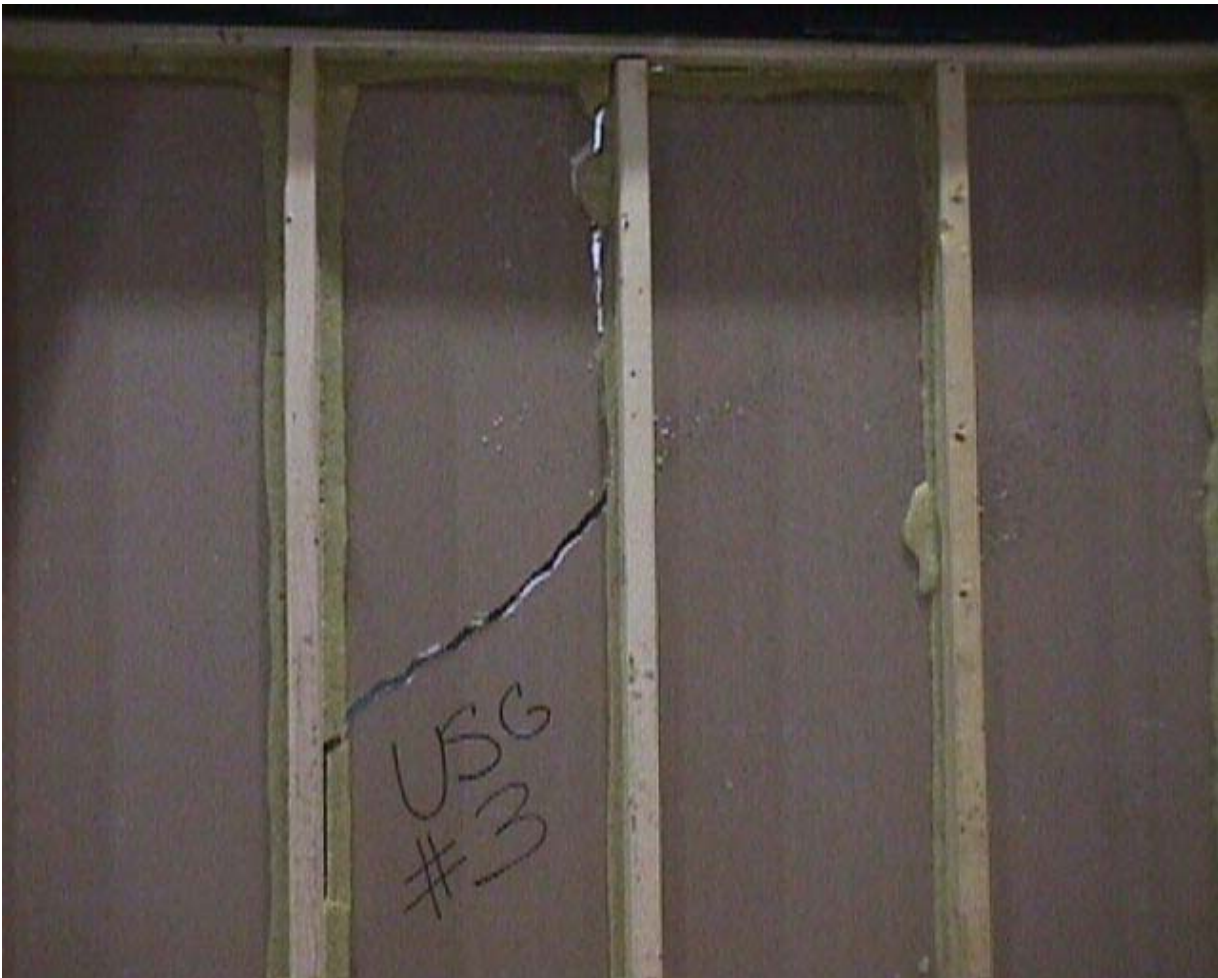
Test No. 3 at Failed Area
