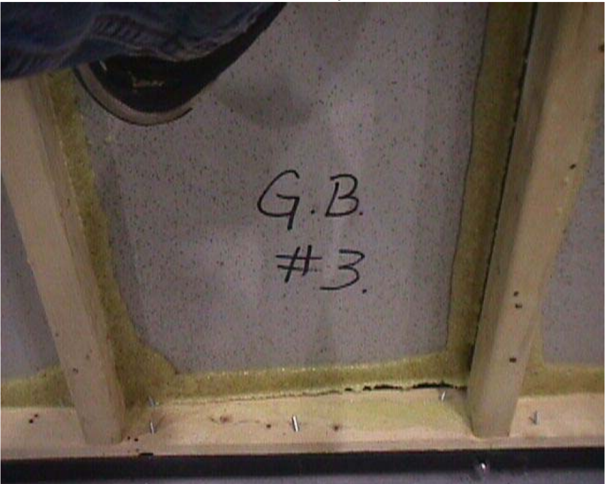
Test No. 3 at Failed Area
