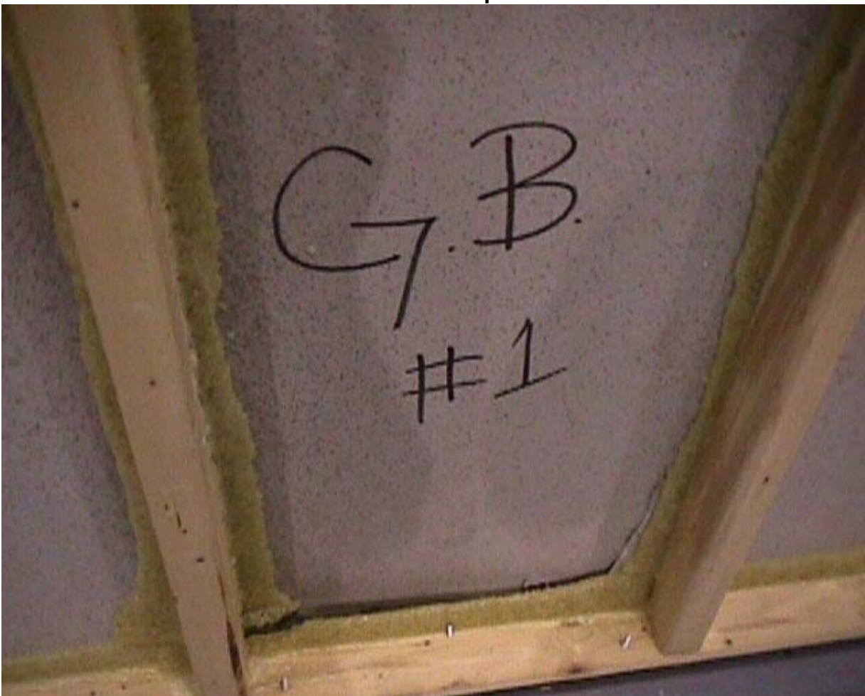
Test No. 1 at Failed Area
