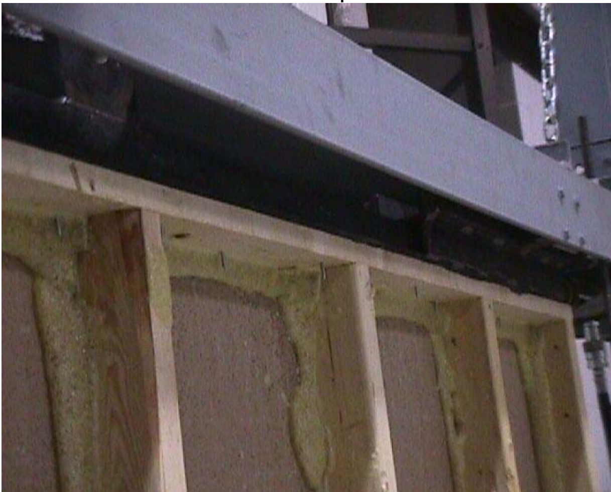
Test No. 2 at Failed Area
